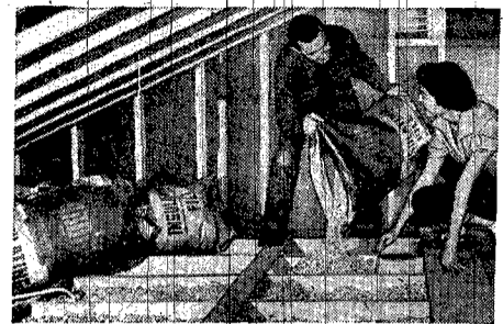
Do-it-yourselfers insulate attic floor joists while she levels material to a 3-inch depth with cardboard rake.
